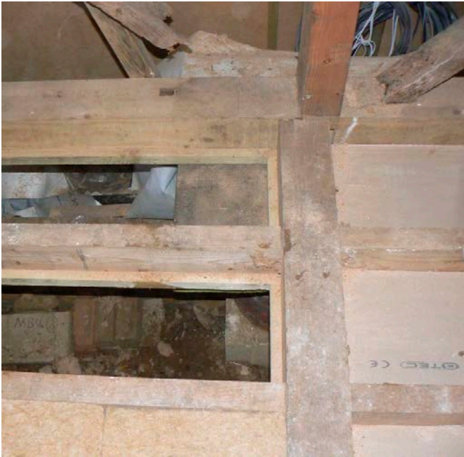
Figure 7: Battens have been added at the sides of the joists to support boarding to carry compressible sheep's wool insulation. © Oxley Conservation
