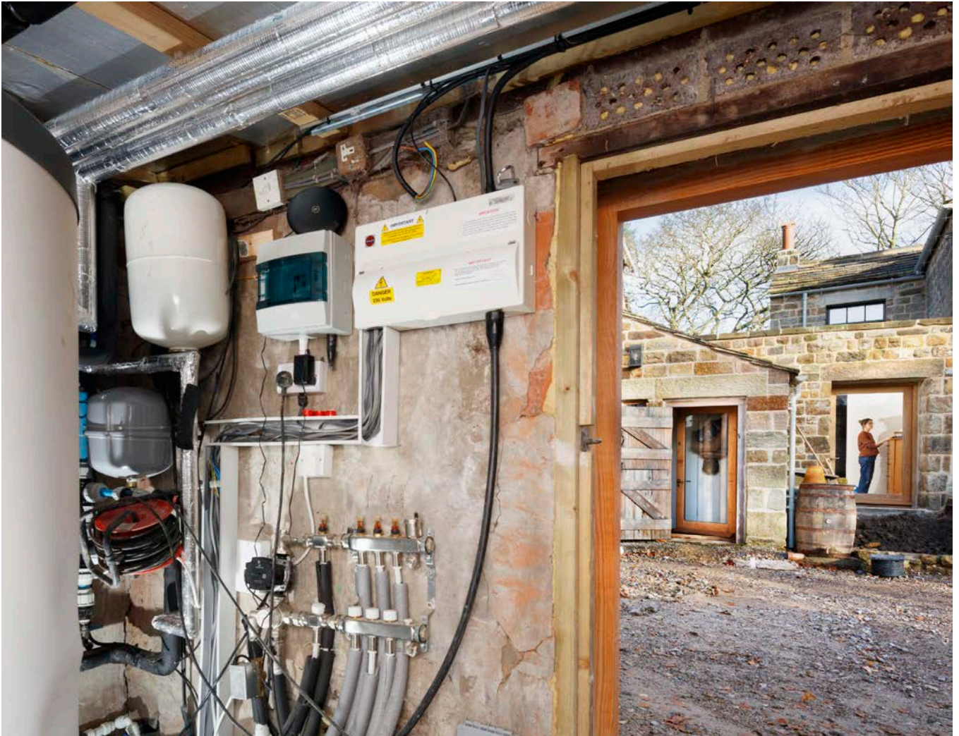
Figure 10: Interior of the outhouse at Hoggerstone Hill Farm, showing the ground source heat pump mechanics, with a view towards the converted farmhouse. © Historic England
